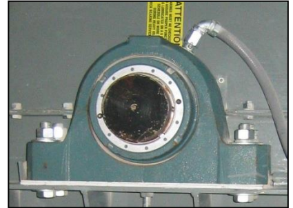
Sensor Installed on Conveyor Bearing
