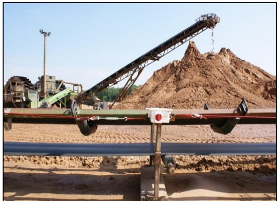
Pullswitch Installed on Open Conveyor at Sand and Gravel Facility
